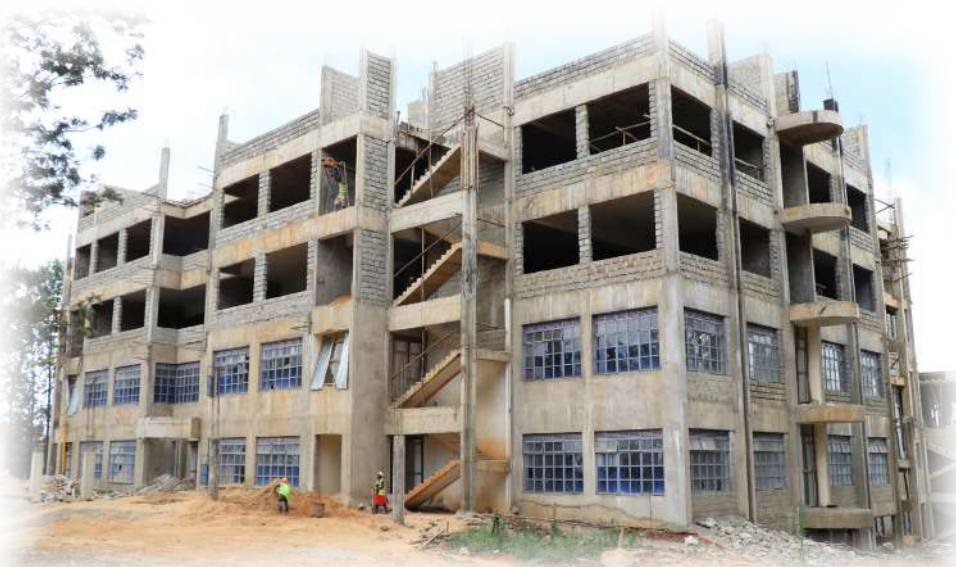
(Top) The artistic impression of the proposed Ultra-Modern Tuition Block. (Bottom) The ongoing construction of the proposed Ultra-Modern Tuition Block.
